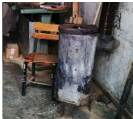
Fig. 6. An example of a stove used for the incineration of waste in Gumushane.
