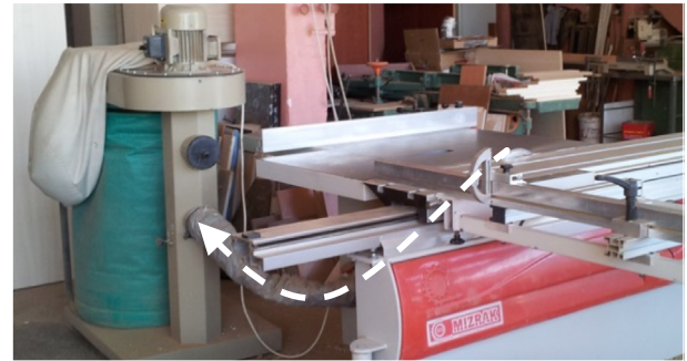
Fig. 4. Example of dust-removal facilities.
